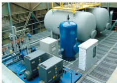
Seongnam Resource Recovery Facility Reconstruction Project Project Owner : Korea District Heating Corporation Contractor : Kenertec Pressure Maintaining System: 1.5m 3 x 2 units
