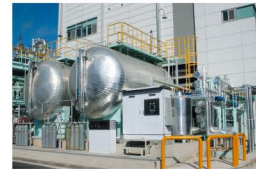
Osan Combined Heat & Power Plant Expansion Project Project Owner : Daesung E&C Cogen Business Unit Contractor : Daesung E&C Pressure Maintaining System: 65m 3 x2 units(2nd)
