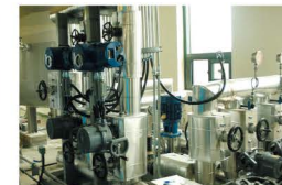
Incheon Hwangchon Heat Exchange Facility Project Owner : Korea Land & Housing Corporation Contractor : KEANGNAM ENETRPRISES LTD Pressure Maintaining System: 12m 3 x 2 units
