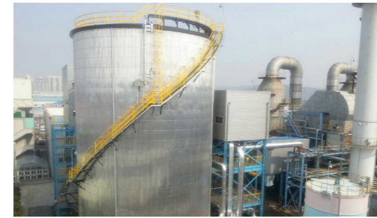
Jeonbuk Iksan District Heating System
